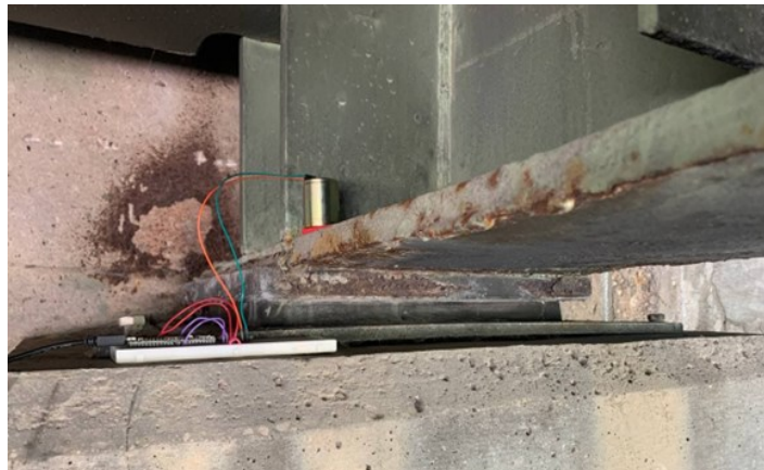
Fig 3.9. The geophone attached location and bearing from the side of view
