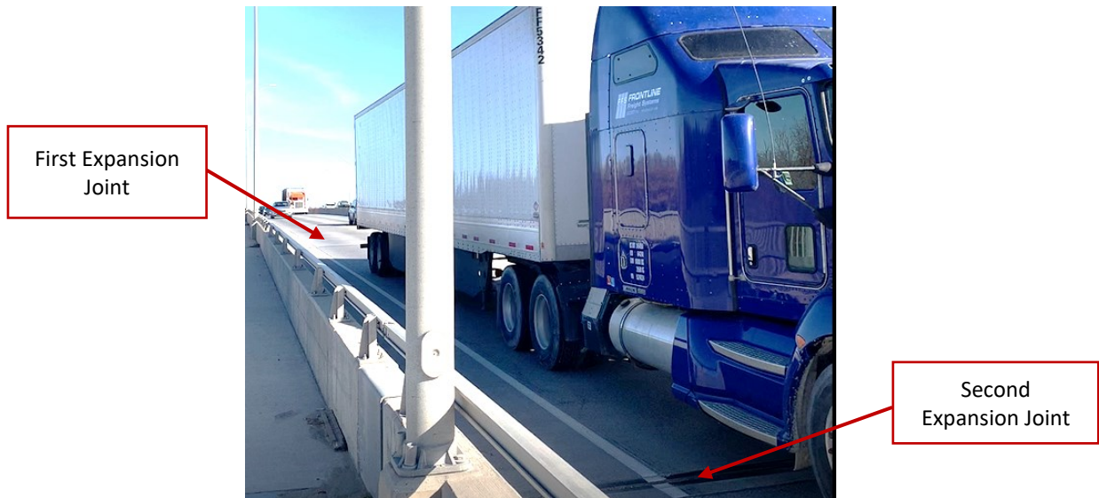
Fig 3.15. The location of two expansion joints can be seen through the attached camera.
