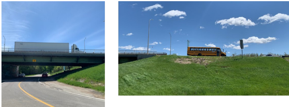
Fig 3.30. The Left Picture is a picture of the bridge from the camera's perspective.
