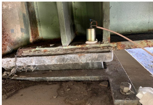
Fig 3.23. The geophone position was attached to the top of the bearing for axle spacing calculations
