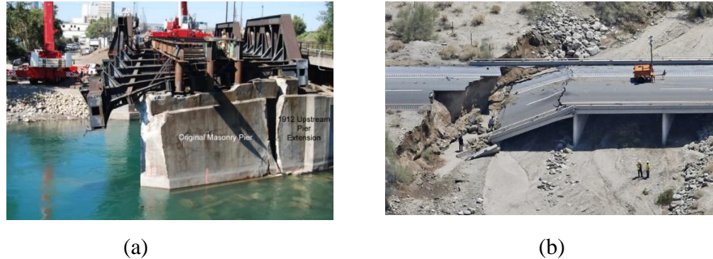
Figure 1-1: Bridge failures due to scour. a) the Bonnybrook bridge in Calgary in 2013 [21]; b) the I-10 bridge in Southern California in 2015 [22]
