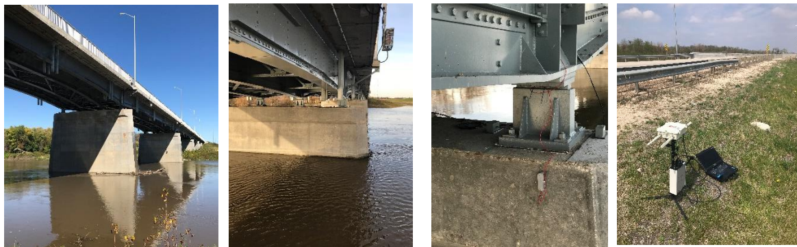
(a) Pier 5 (b) close view of Pier 5 (c) installed sensor (d) data acquisition
