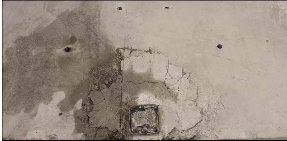
a) Slab top surface at failure
