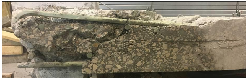
d) Internal cracking
