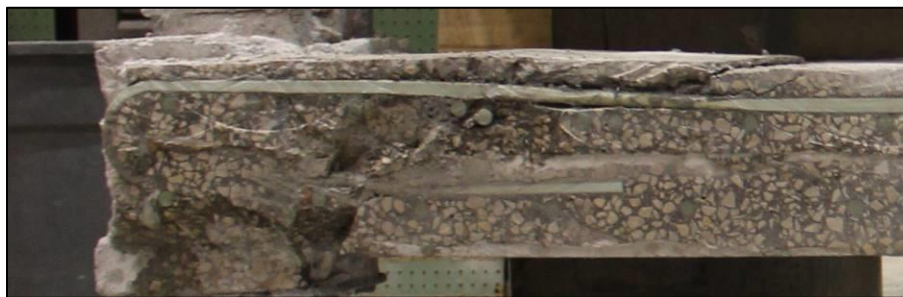
d) Internal cracking
