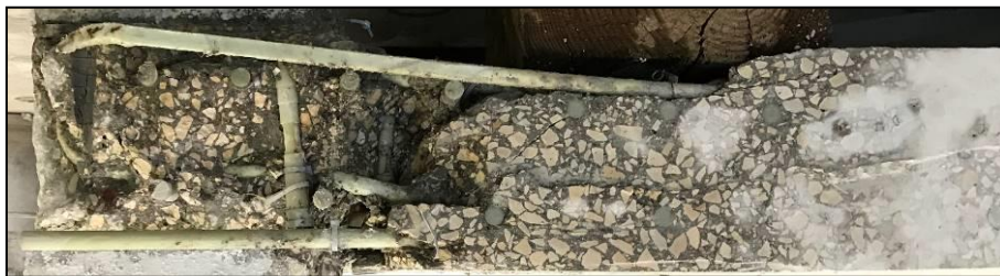
d) Internal cracking
