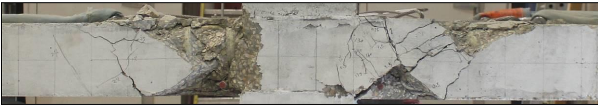
c) Slab free edge after 3.50% drift ratio (at failure)
