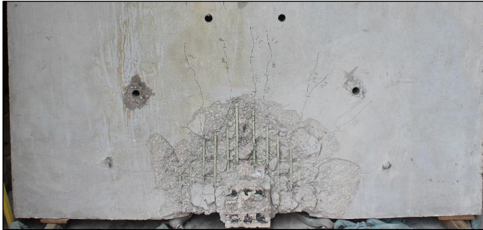
a) Slab top surface at failure
