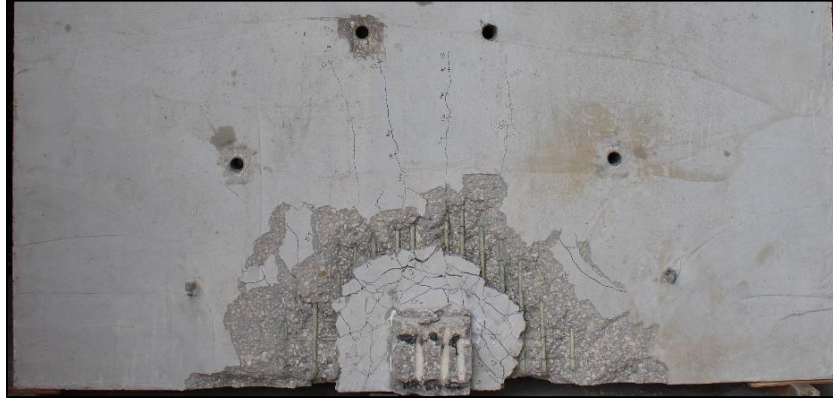
a) Slab top surface at failure
