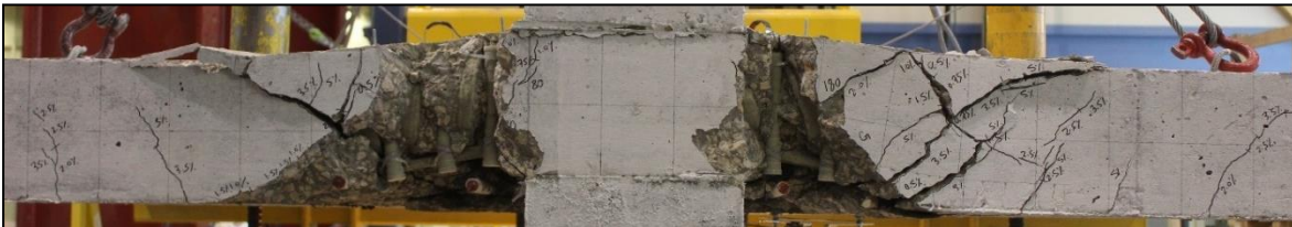
c) Slab free edge after 6.50% drift ratio (at failure)
