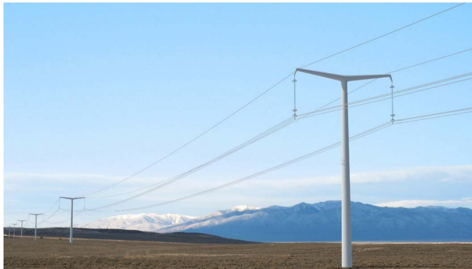
Figure 3-13 Modern pole tower structure for HVDC Transmission (courtesy of Bystrup)
