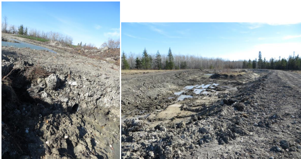
Figure 1. It's a little difficult to see, but the pond (left) is connected to the channel in the left of the picture by a culvert (in the bottom right quadrant). The constructed but still empty wetland is pictured right.
