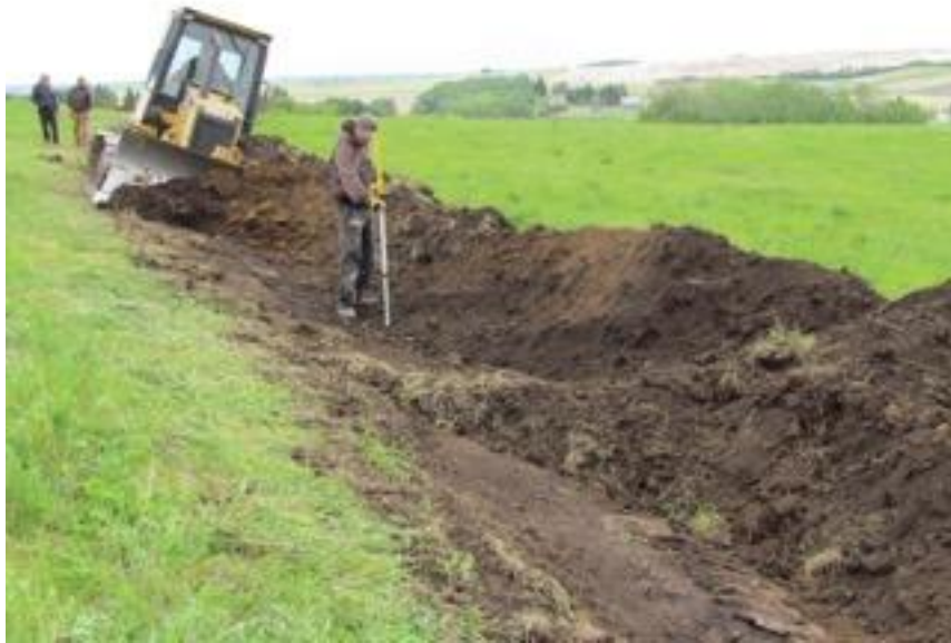
Figure 17. Ensuring the level is accurate during construction of the top swale (photo courtesy of Takota Coen).
