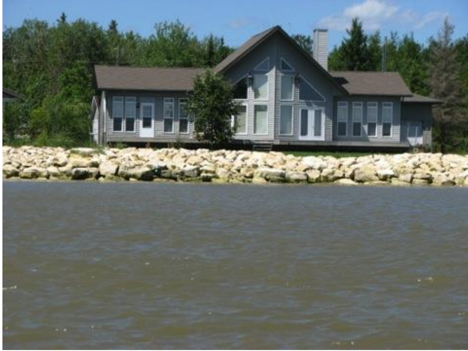
Modification – recent rip-rap erosion
