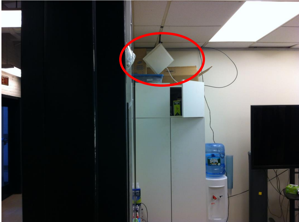
Figure 6.3 Antenna in Room 35-205
