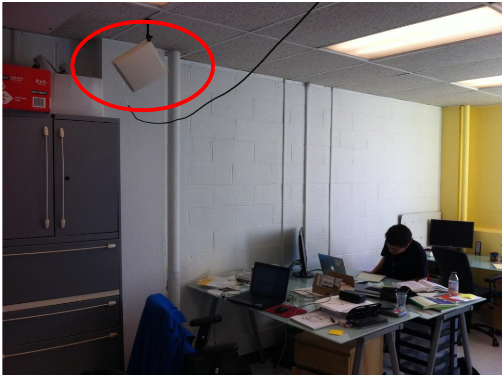
Figure 6.2 Antenna in Room 35-203
