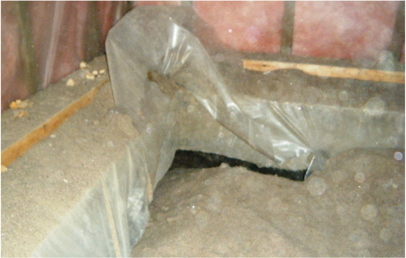
Figure 6: Unstable sub-foundation. Note cavity below footing
