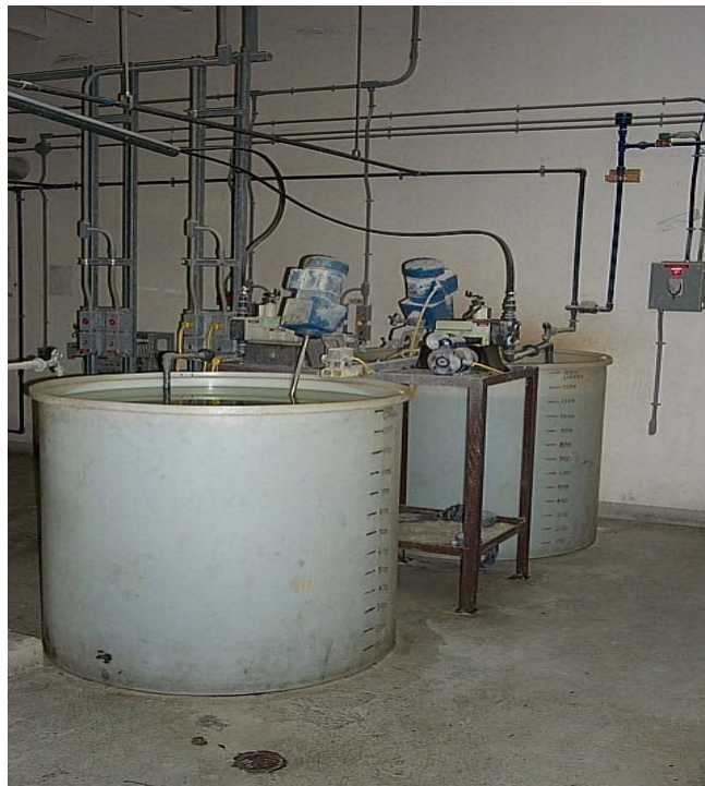
Figure E-3 Alum coagulant feeding facility at the Split Lake WTP
