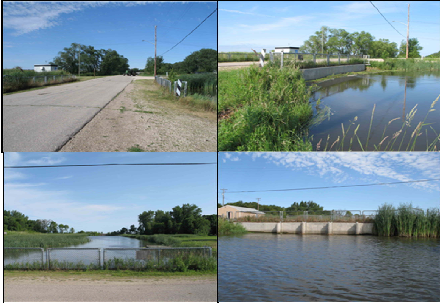
Figure 3.7 Photograph of Delta Channel Bridge on Delta Channel taken in July 2005. Pictures (top left) view west of the bridge looking east at the bridge, (top right) view of the bridge looking southwest, (bottom left) view from the bridge looking north down Delta Channel, and (bottom right) view from Delta Channel looking north at the bridge.
